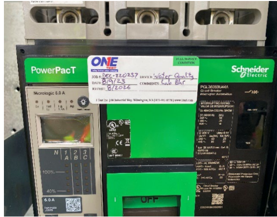
Typical 600 Amp Breaker
